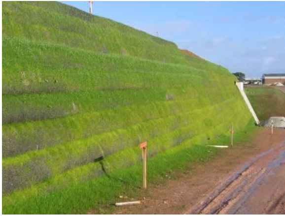
Figure 21 Vegetated 'green' finish [9]
