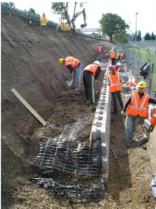
Figure 20 The chosen Geosystem should be appropriate for the available working space and any other restrictions [11]
