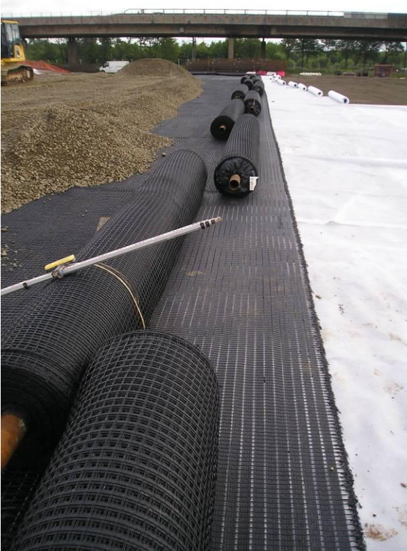
Figure 25 M6 Extension, Guardsmill; used high strength, low strain uni-axial geogrids to construct embankments [4]
