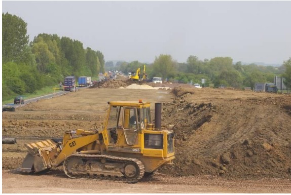
Figure 39 An appreciation of the materials, methods of construction and site constraints can be invaluable in the selection of Geosystems [5]
