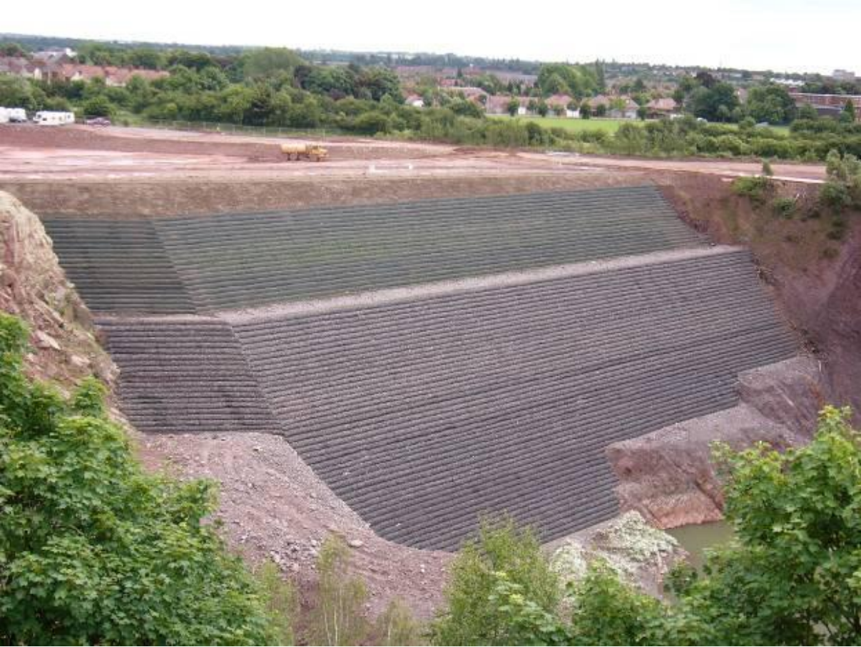
Figure 23 Midland Quarry; Nuneaton. Arguably the largest Geosystem structure in the UK. Formed of reinforced soil utilising a blend of site won materials and an imported 'waste' foundry sand as the backfill [16]
