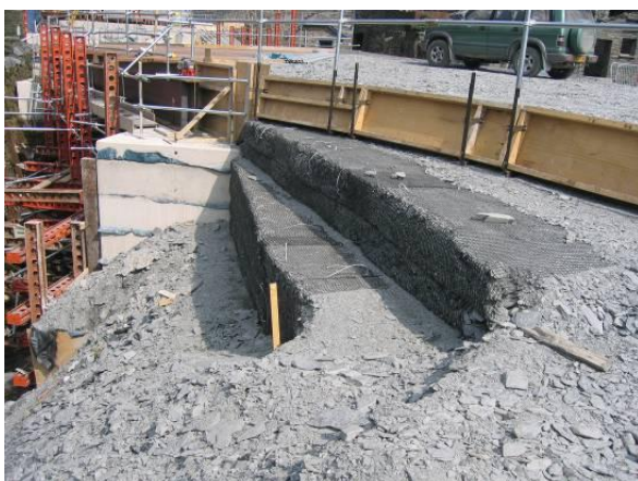
Figure 31 Blaneau Ffestiniogg, Wales. Temporary road diversion formed from wrap around reinforced soil slopes utilising locally available waste slate material as a backfill [5]
