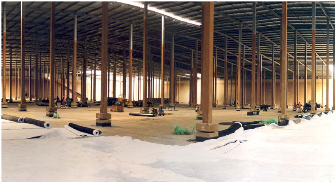
Fig 2. A large water storage basin with a fixed roof structure with hundreds of columns.
