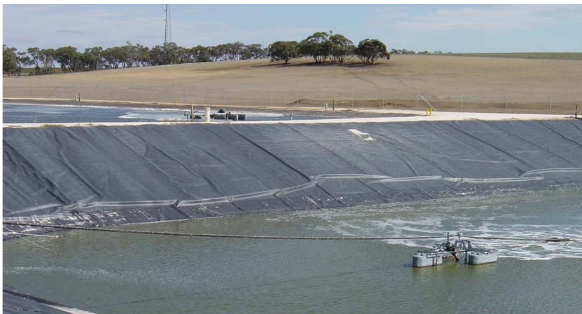
Fig 8. HDPE Lagoon with Floating surface aerators
