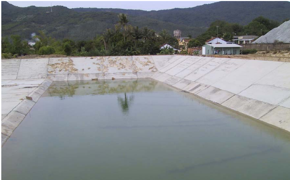
Fig 1. A water storage facility based on a GCL liner with concrete covering.
