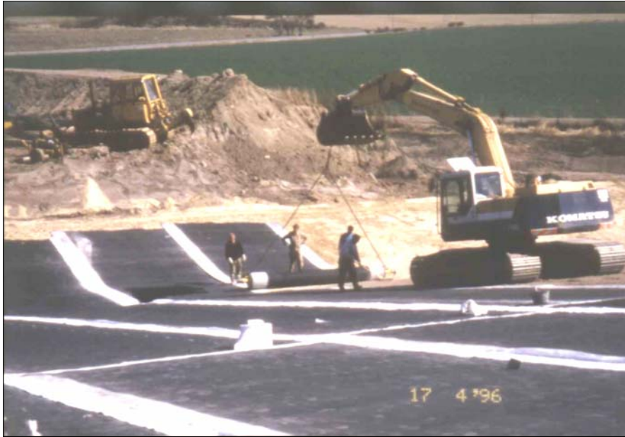
Fig. 2: Installation of the geosynthetic clay liner (GCL) as part of a geosynthetic cover system at the landfill Neu Wulmstorf near Hamburg, Germany, 1996/97
